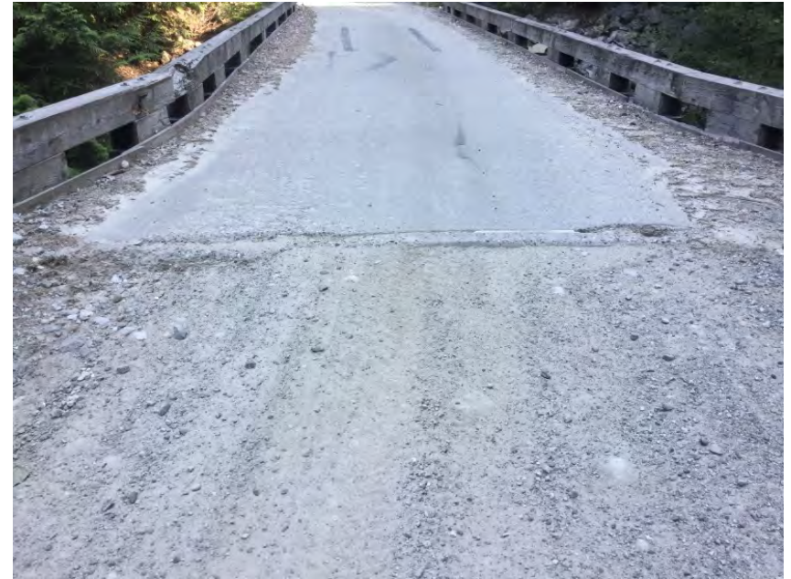
Left approach ballast wall and deck damage
