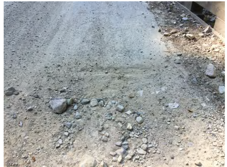
Right approach concrete damage
