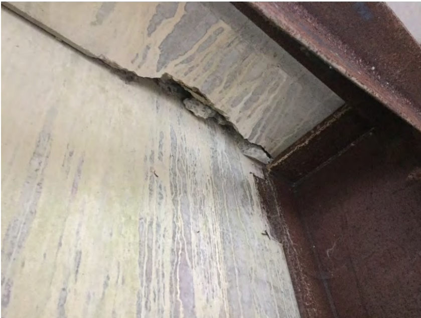
Right approach deck panel damage
