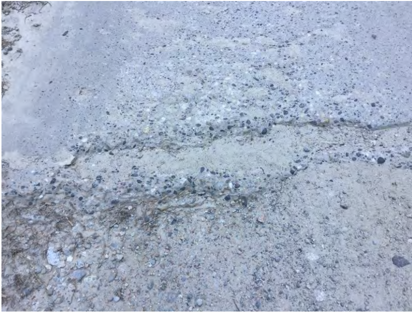
Left approach concrete damage
