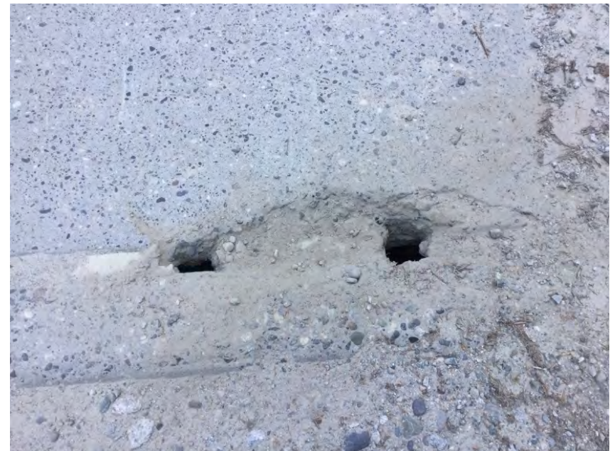
Left approach concrete damage
